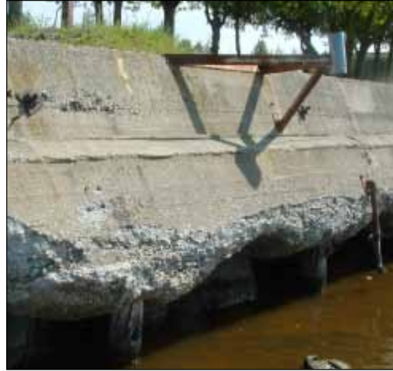
Figure 2: Concrete Structure Problems on Lake Michigan.
