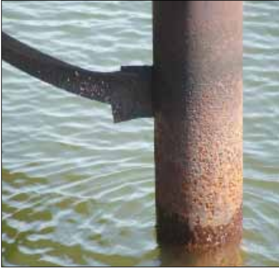
Figure 1: Steel Corrosion on Lake Superior.
