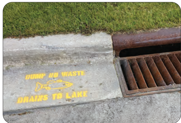
Storm drain stencil at Harbor Centre Marina. Photo credit: Julia Noordyk, Wisconsin Sea Grant.
