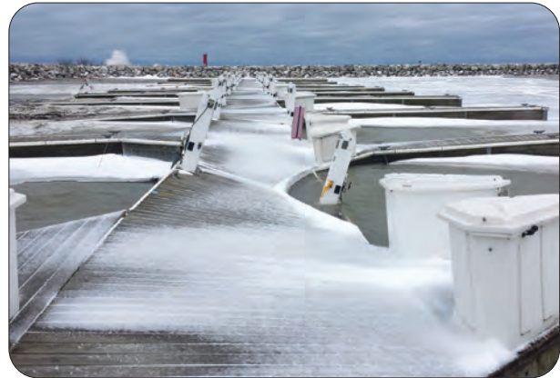
Ice damage at Harbor Centre Marina. Photo credit: Matt Bauer, F3 Marina.
