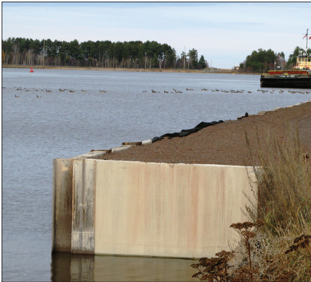
Figure 12: A new wall in front of a failed timber structure (Chad Scott-AMI Consulting Engineers).
