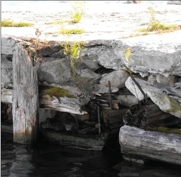
Figure 4: Timber structure rot (Gene Clark/UW Sea Grant Institute).
