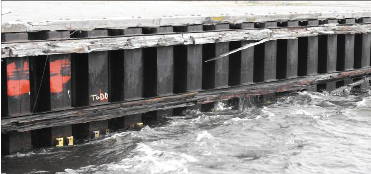
Figure 8: Timber ice abrasion damage (Gene Clark/UW Sea Grant Institute).
