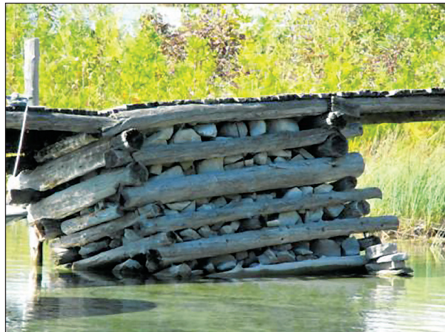
Figure 7: Timber crib settlement failure (Gene Clark/UW Sea Grant Institute).
