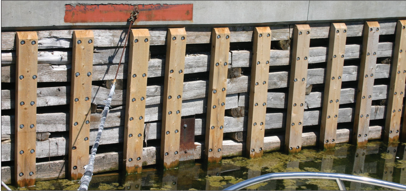
Figure 11: A failed timber reinforcement section (Larry Ryan-Baird).
