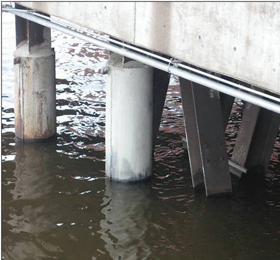
Figure 13: Steel jacket option shown on steel pile (Gene Clark/UW Sea Grant Institute).
