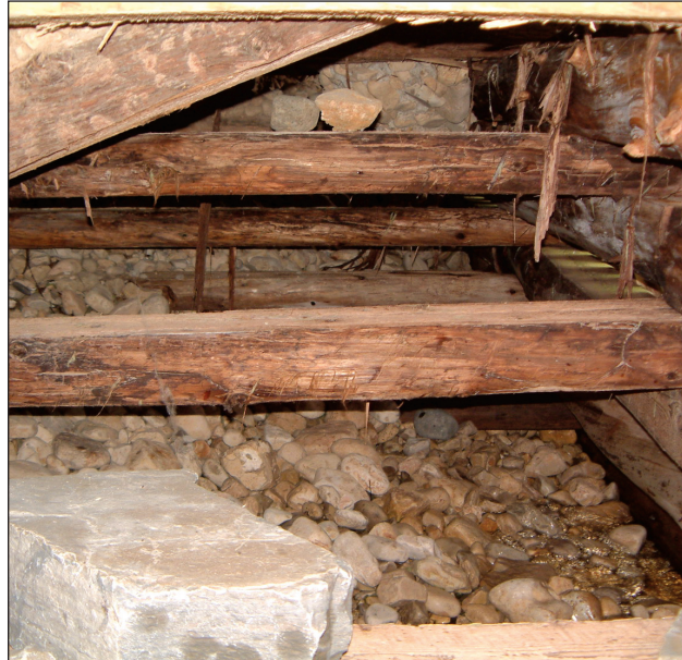
Figure 6: Timber crib with interior rock loss (Bill Brose-SmithGroupJJR).
