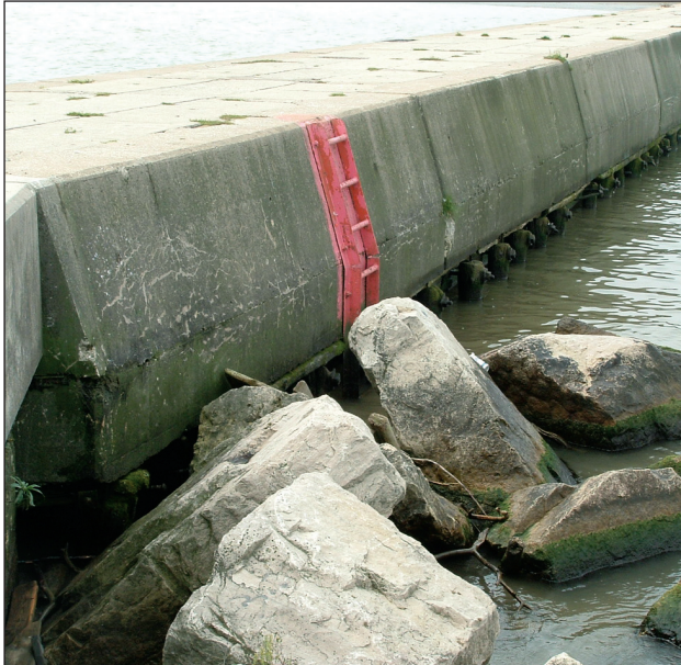
Figure 1: A typical U.S. Army Corps of Engineers breakwater section (Gene Clark/UW Sea Grant Institute).
