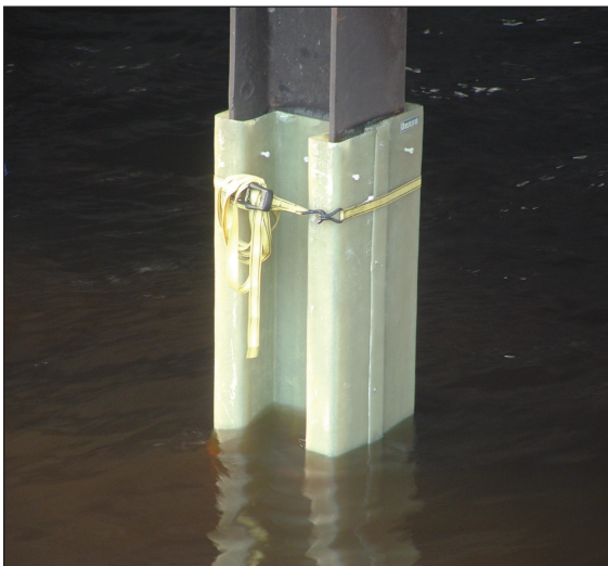
Figure 14: Fiberglass jacket option shown on steel H-pile (Gene Clark/UW Sea Grant Institute).
