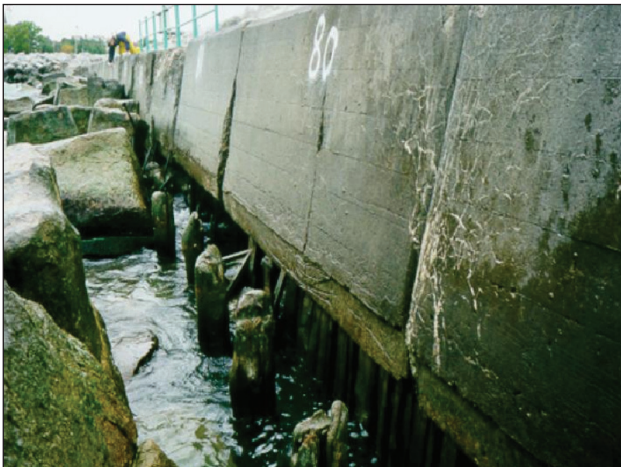
Figure 5: Timber piling rotting at the water surface (Larry Ryan-Baird).
