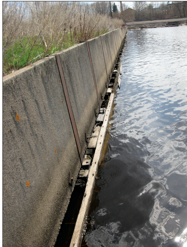
Figure 10: New wall constructed on top of failed timber crib (Chad Scott-AMI Consulting Engineers).
