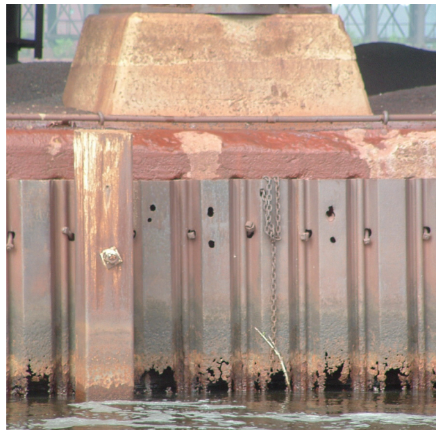
Widespread corrosion at Hancock, Michigan, (above) and Canadian National docks, Duluth, Minnesota (below)
