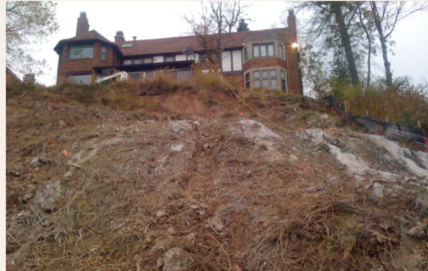
Before Before stabilization, the bluff was failing very close the residence, indicated by the steep unvegetated slope close to the home. Marek Landscaping
