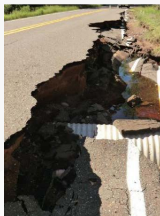
Culvert damaged in 2016 flood, Ashland County
