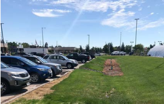
Parking lot bioretention, city of Superior
