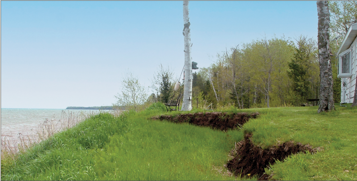
CLOCKWISE FROM TOP Horizontal ground cracks at the top of the bluff that preceded a slope failure. Gene Clark
