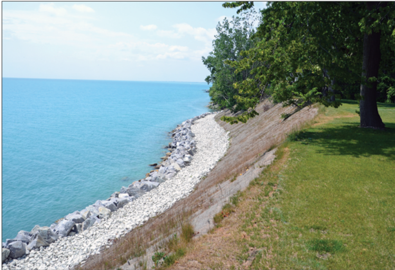
Before and after a cut-and-fill bluff regrading project with shore protection. Adam Bechle
