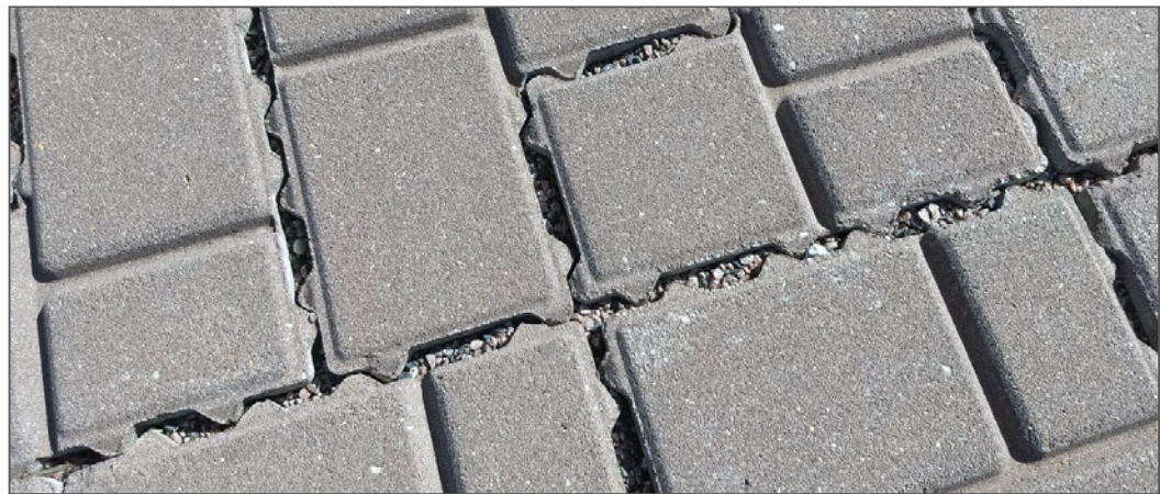
Permeable pavers used for bluff-top parking spots. Adam Bechle
