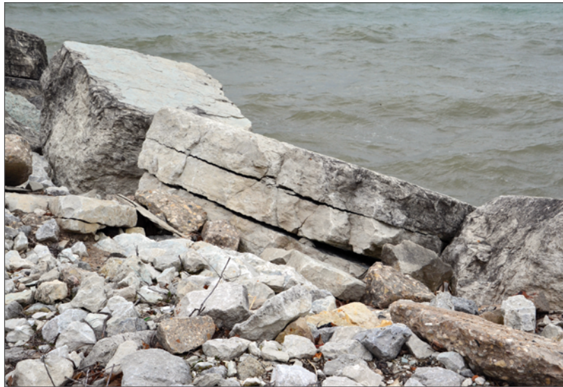
TOP Displaced armor stone has exposed the underlying filter layer to wave forces. Adam Bechle BELOW Cracked armor stone has split into smaller pieces. Adam Bechle
