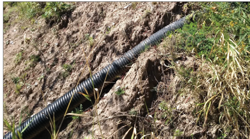
Drainage pipe carrying water to the base of the bluff. The pipe is located in a gully that surface water runoff previously eroded into the bluff. Adam Bechle
