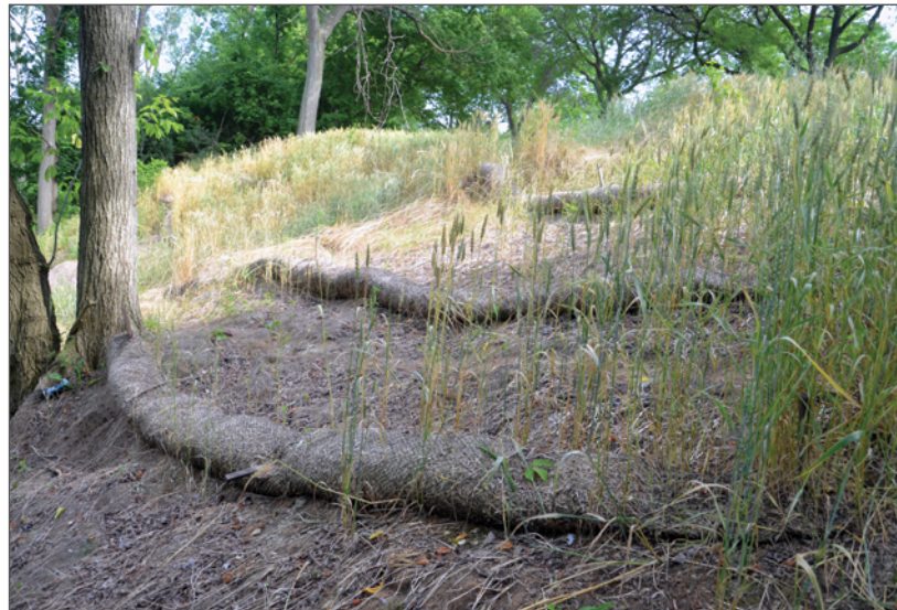
Coir logs staked into the bluff to slow surface water flow down the bluff face and help vegetation establish. Lydia Salus
