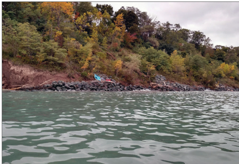
LEFT Flanking around the unprotected end of the revetment has led to accelerated erosion. Chin Wu RIGHT Overtopping of this revetment has led to erosion on the back side of the armor stone. Adam Bechle
